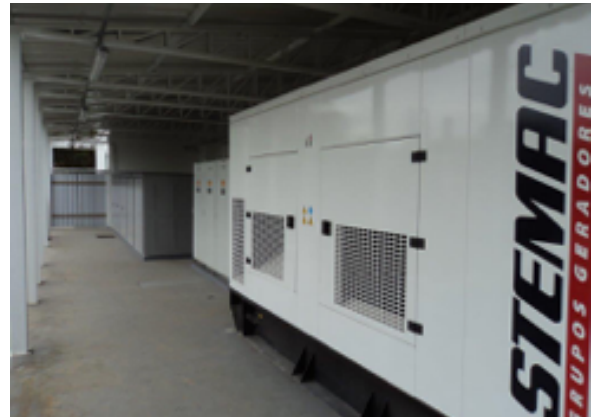
Figure 14 - New Radiopharmacy Center electrical supply cabin
