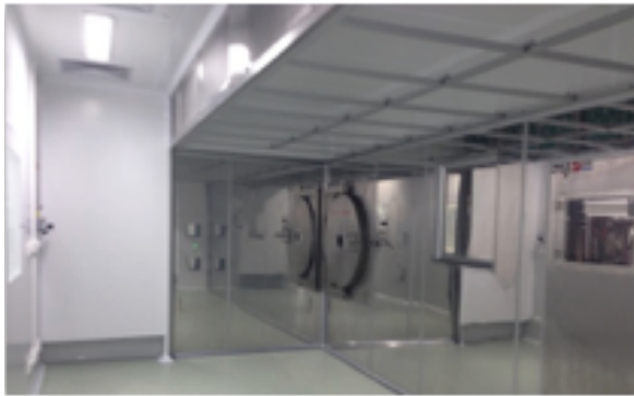
Figure 12 - New freeze dryers
